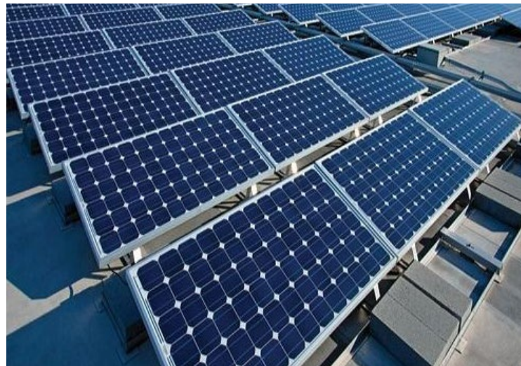
ROOFTOP PHOTOVOLTAIC ARRAY
